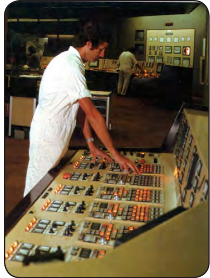
Fig. 2: Gladstone Power Station plant control room ( QEGB Newsline , March 1982)
